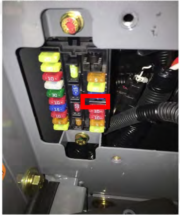
TL8 Uninstalled Fuse Example Cover Open
