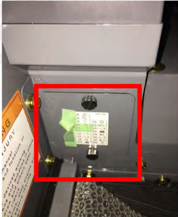
TL10 TL12 Uninstalled Fuse Example
