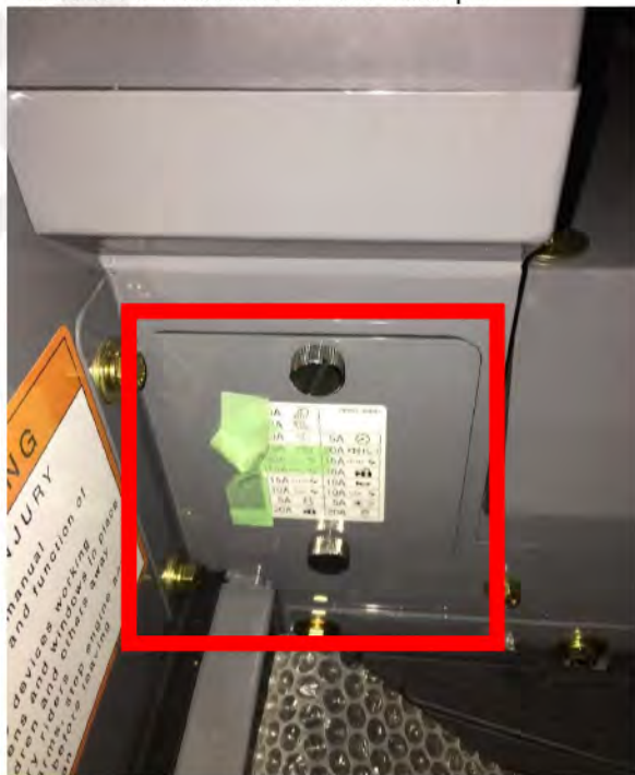
TL10 TL12 Uninstalled Fuse Example
